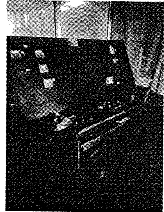
TEST BENCH FOR TRANSFORMERS
